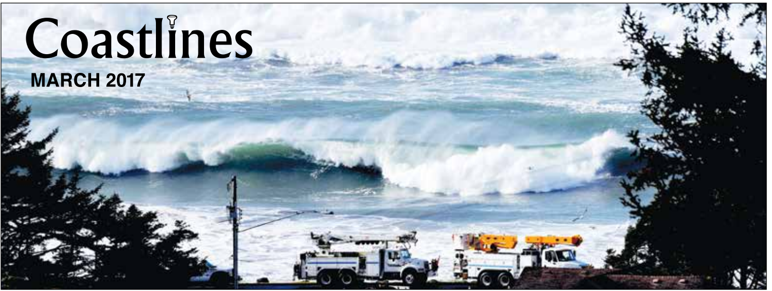
Our 30' digger derrick truck (center) and 30' bucket truck are dwarfed by huge winter waves on the Pacific. Photo ©Ken Gagne
