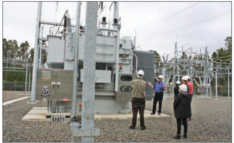
Central Lincoln Engineering Manager Bruce Lovelin (blue shirt) proudly leads a tour of the new substation.
