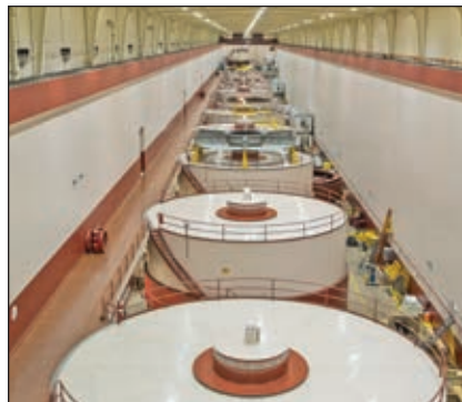
The row of generators inside the powerhouse at the Chief Joseph Dam.
