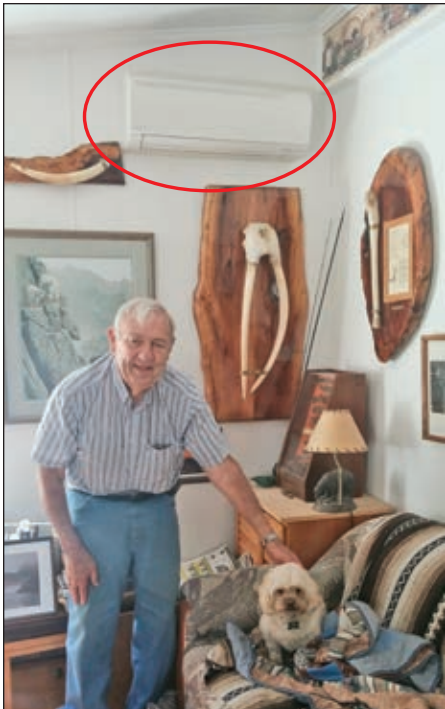
Jerry Christean and Charlie appreciate the comfort of their ductless heat pump (red circle above)
