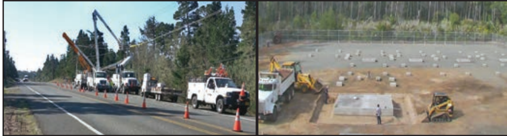
(left) Drivers on Highway 101 between Heceta Beach Road and 27th Street in Florence will need to watch for traffic cones, trucks, and linemen working on the shoulder of the highway. (right) An aerial view of the work underway at our new substation in the Pacific View Industrial Park in Florence.
